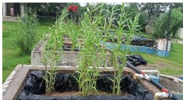
Figure 4: Typical picture showing SSVF CWs Beds
